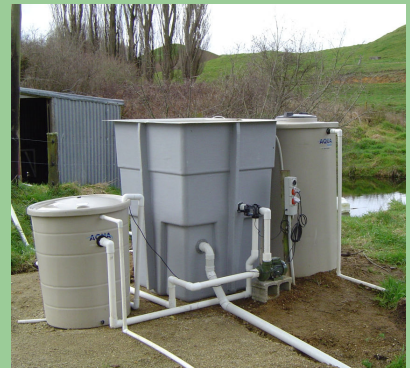
TURBIDITY REDUCTION SYSTEM FOR POND/DAM WATER
