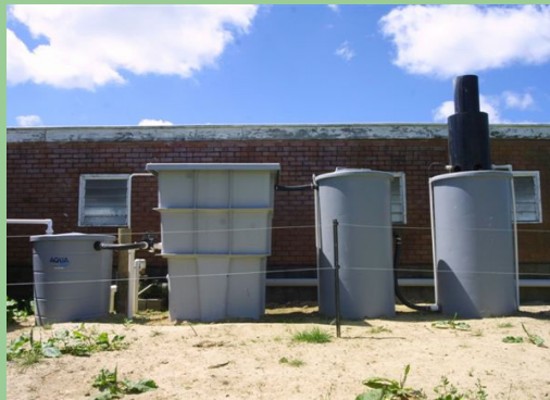
IRON & MANGANESE SYSTEM FOR BORE WATER
